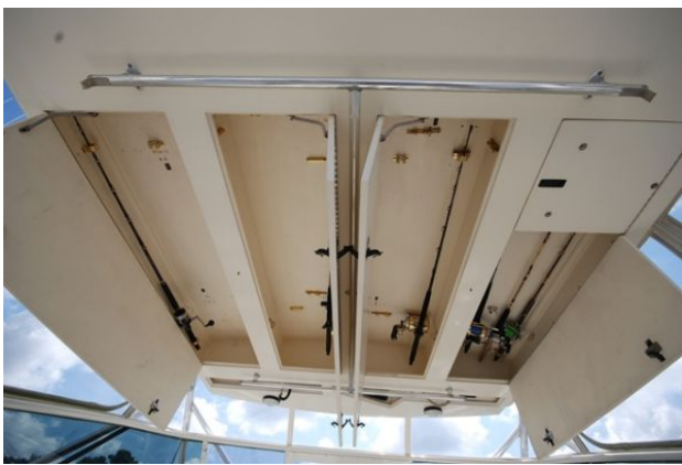
OVERHEAD ROD STORAGE
