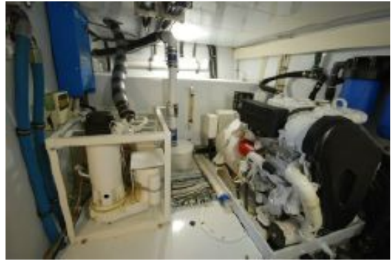
> Chipper and Genset 2 / Pump Room
