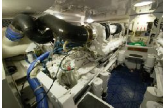
> Engine Room -Port
