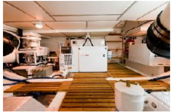
ENGINE ROOM VIEW 4
