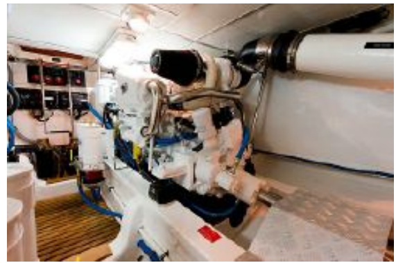
ENGINE ROOM VIEW 2
