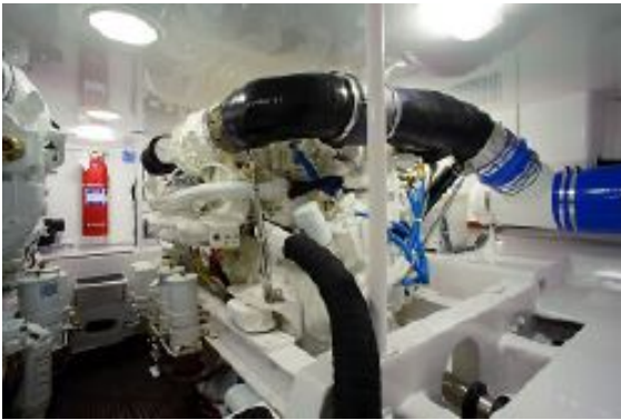
Engine Room View 2
