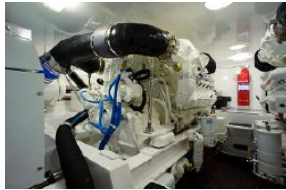
Engine Room View 3
